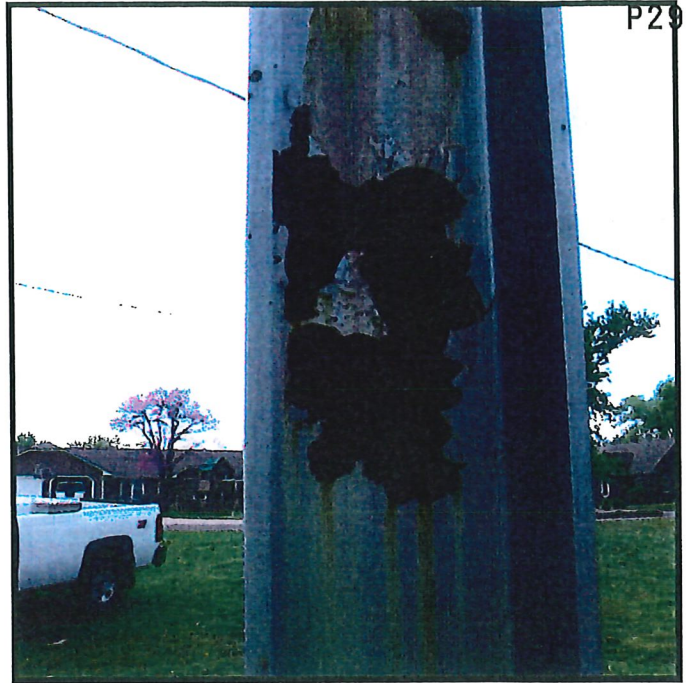
Peeling of existing coatings and corrosion present.
