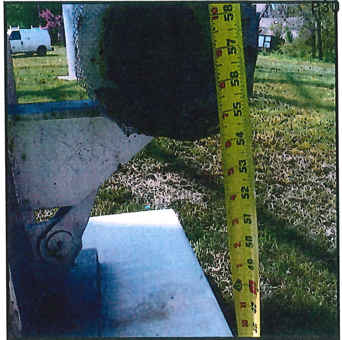
Existing overflow pipe is 54" from ground. AWWA/ KDHE standards state that overflow should be 12-24" from ground with screen and flapper.
