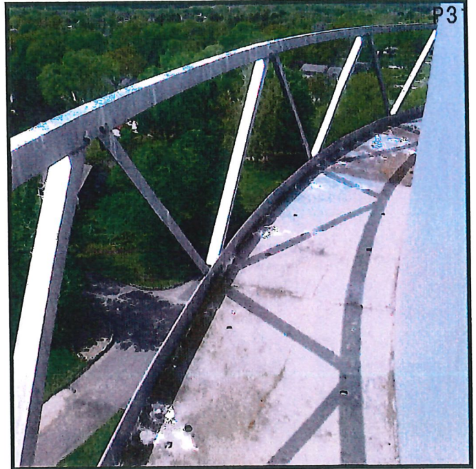
Openings at handrail exceed OSHA measurement standards (max round 19"). Recommend installing a "mid-rail" to meet OSHA standard.
