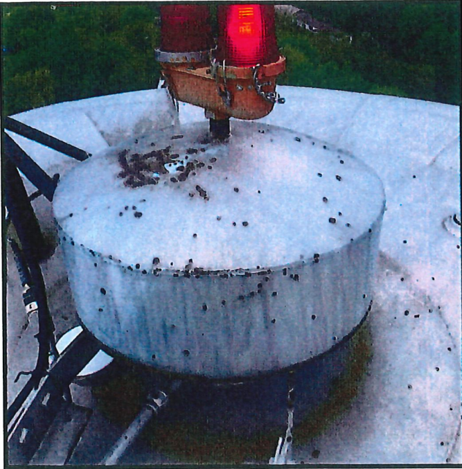
Roof vent should be replaced to meet AWWA/ KDHE "fail-safe" standards.
