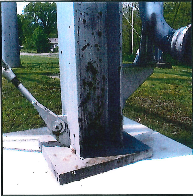
Corrosion at tank leg. Note the overflow pipe attached to leg.
