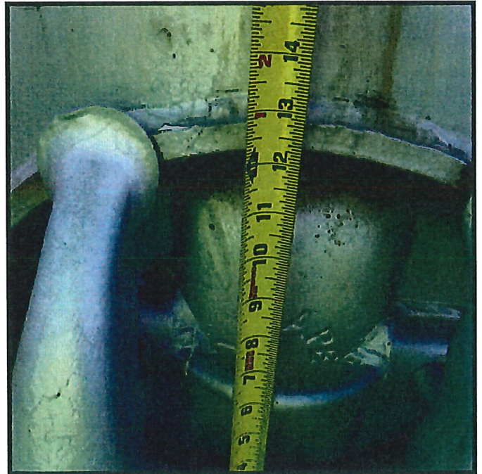
OSHA standards state that opening needs to be 24" diameter minimum.
