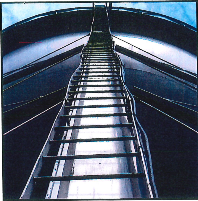
No safety climb device is present at ladder. Recommend to install cable style safety climb device.
