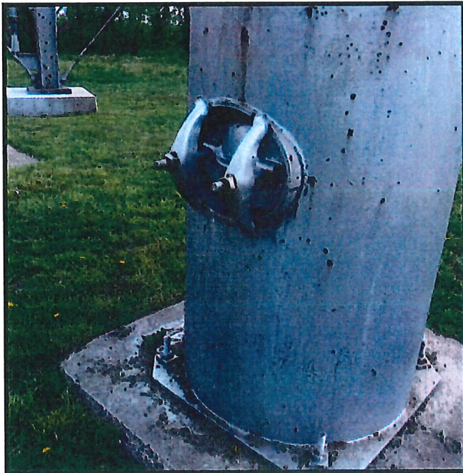
Existing non-compliant riser manway.
